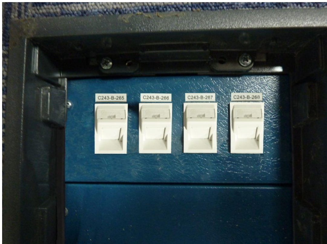
Fig 4.3: Example of the layout of a floor box, showing the LJ6C angled fascia sockets pointing towards the middle of the floor box.
