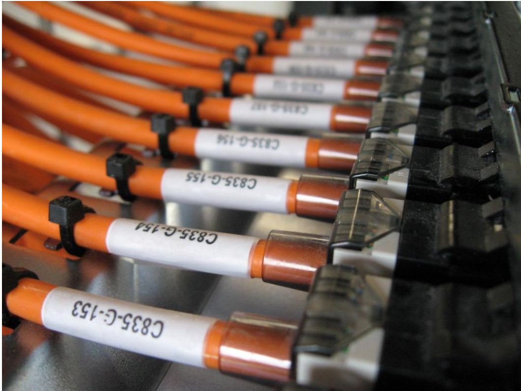
Fig 6.1: Example of cable label on UTP at the back of the patch panel
