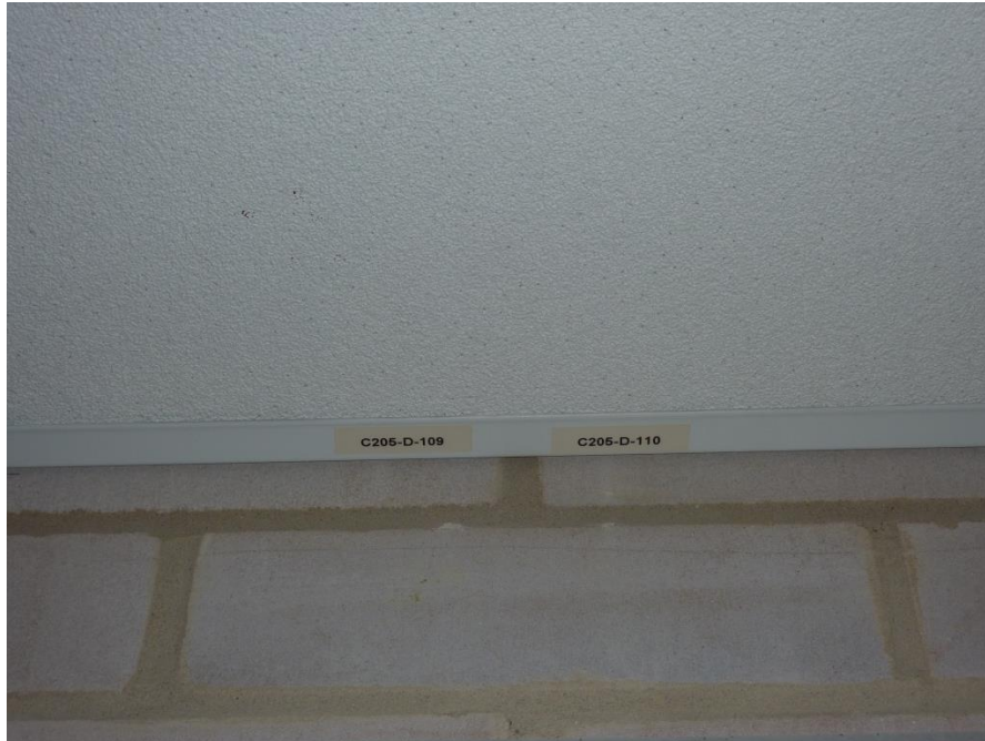
Figure 9-3: Example of labelling below suspended ceiling
