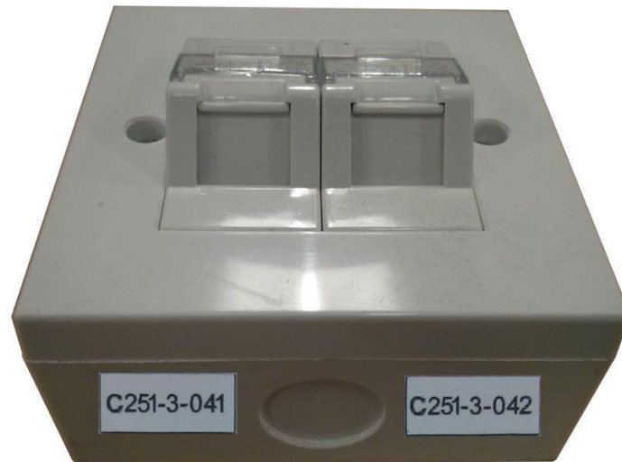
Figure 9-2: Example of labelling position on a high level patch panel box, so it is visible from below
