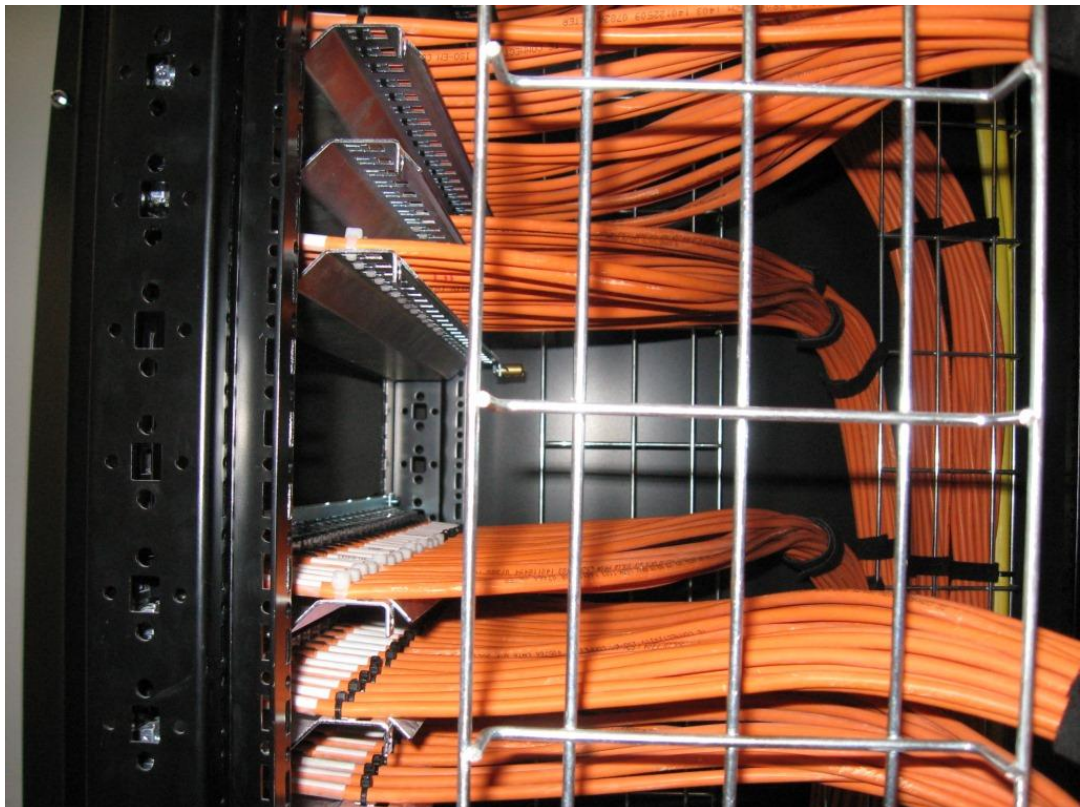
Fig 8-1: Shows how network cable should be installed to avoid intruding into space used for network equipment
