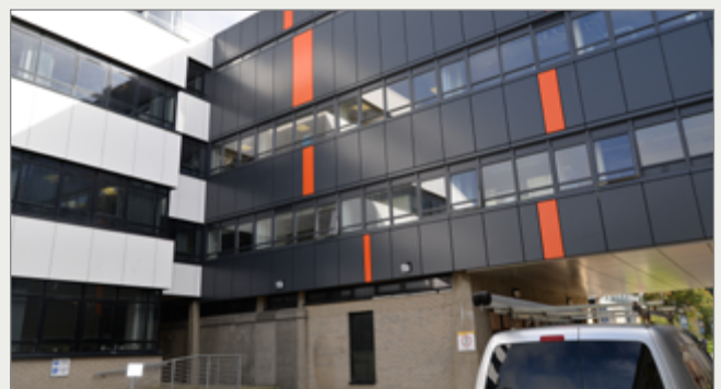
Cledwyn bridge and spur after the addition of insulated cladding, installation of modern double glazed window units and replacement of roof surface.
